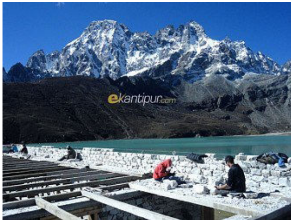
Photo captured during an autumn afternoon, workers are seen busy in the construction of a hotel near Gokyo Lake at the altitude of 4800 meter in the Everest region.
